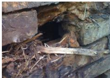
Figure 19 - Liner found to be in contact with chimney brickwork
