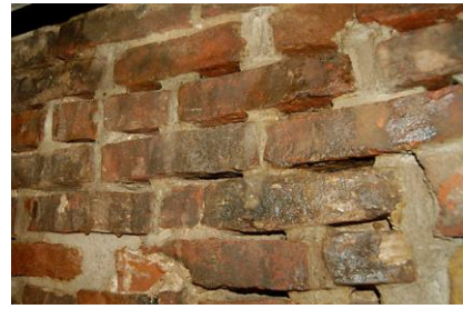
Figure 16 - Imperfect mortar in brickwork
