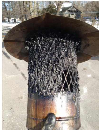
Figure 18 - Tared up chimney bird guard
